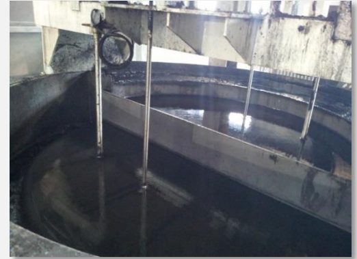
Anhui Huaibei Liudong coal preparation plant
